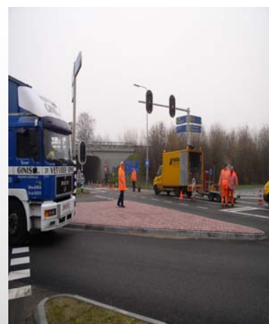
Installation of a backup power system
