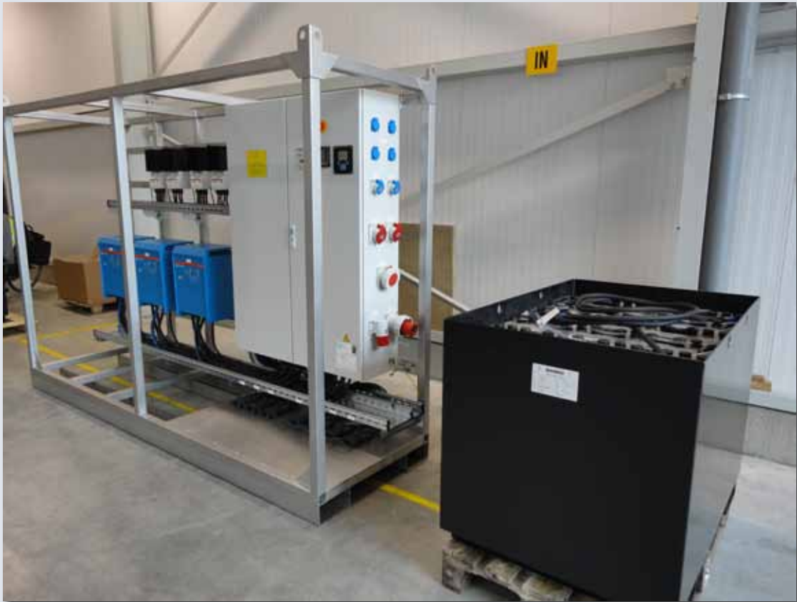
Photo 4: The three Quattro's are connected to the two enormous battery sets.
