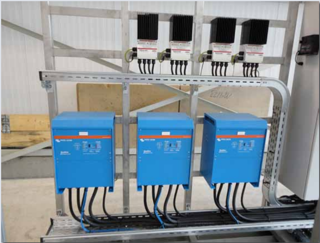
Photo 1: Three Victron Quatro's at the center of the solar energy system.
